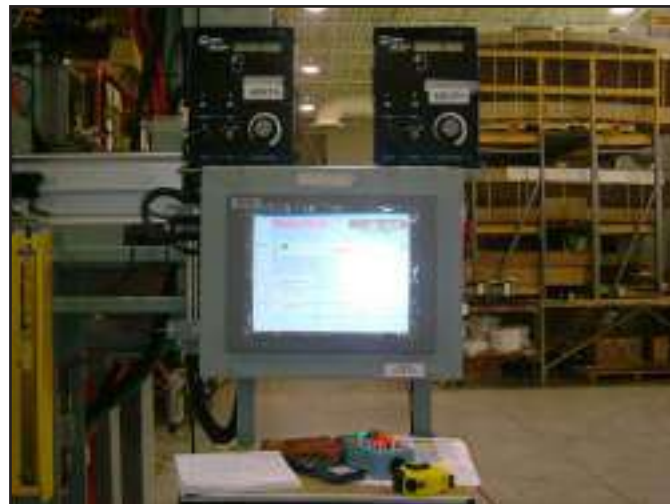
Touch screen industrial PC utilizing Citect HMI software.
